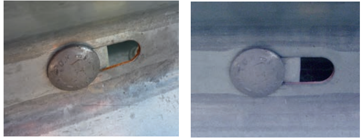
Safety barrier by Mieres Tubos/Grupo Condesa coated in Magnelis® ZM310 (steel thickness 3 mm). Exposure was started outdoors in September 2011 (left). Note the self-healing effect on the perforations in October 2013 (right).
